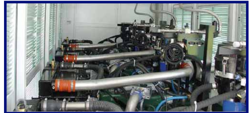
Interior View of HEC 250 kW H 2 Genset
