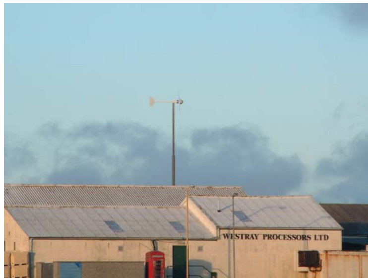
Figure 3 – 6kW turbine at local shellfish co-operative.
